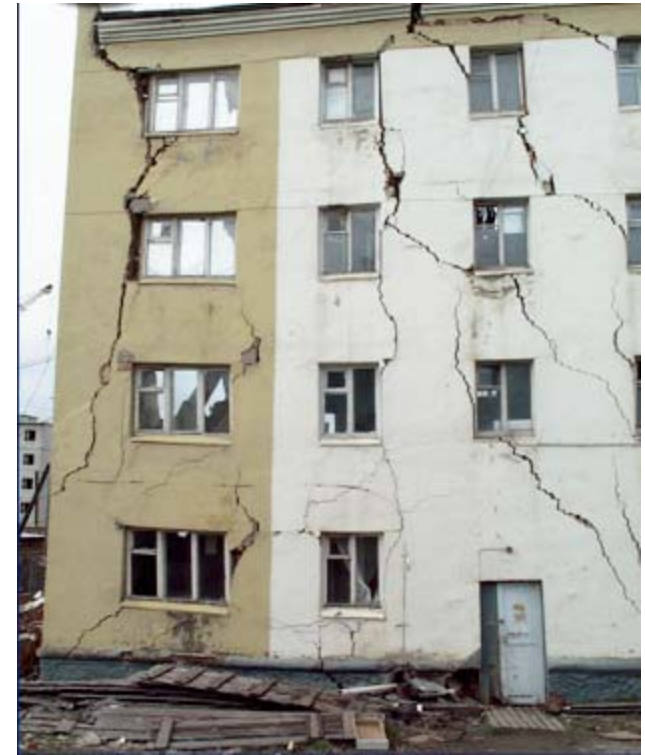
Damage to a Russian Building from melting permafrost
